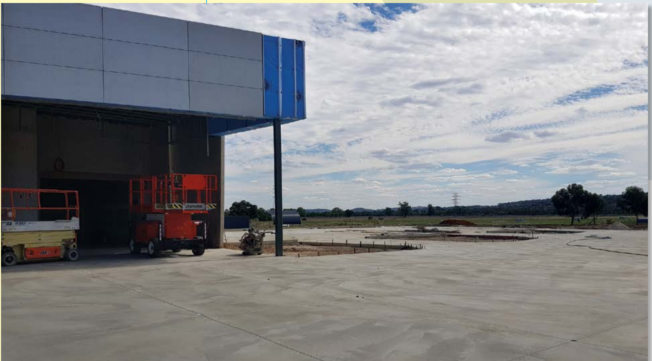
New ACTA Club House and Function Centre showing the expanse of concrete
