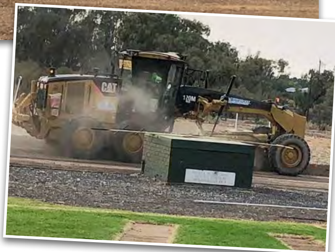
Right: Wads, lead and old clays needed to be removed to prepare the surface
