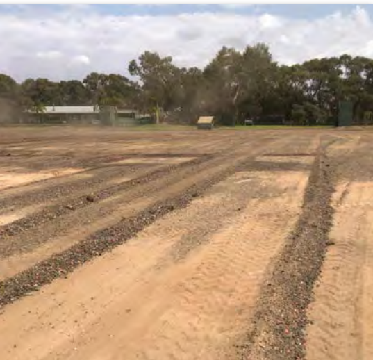
The whole shot area was graded/levelled with a slope fall of 1.5m from around the trap houses to where the curtains were being installed some 80m away
